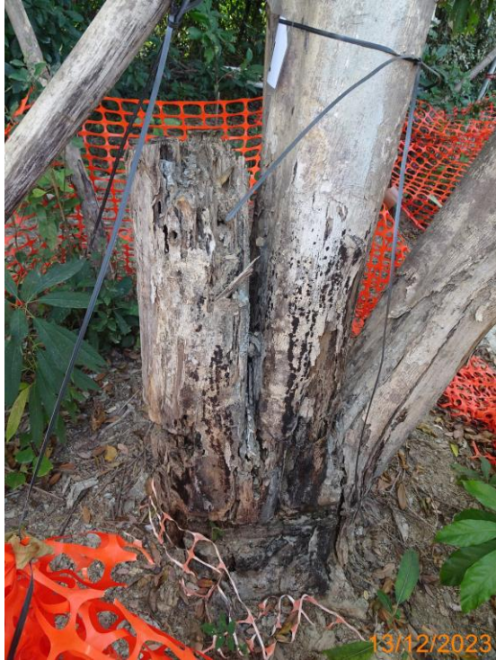
9: U041_ Wood damage at trunk union
