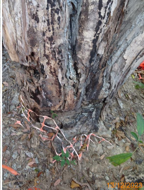
10: U041_ Wood damaged by termite
