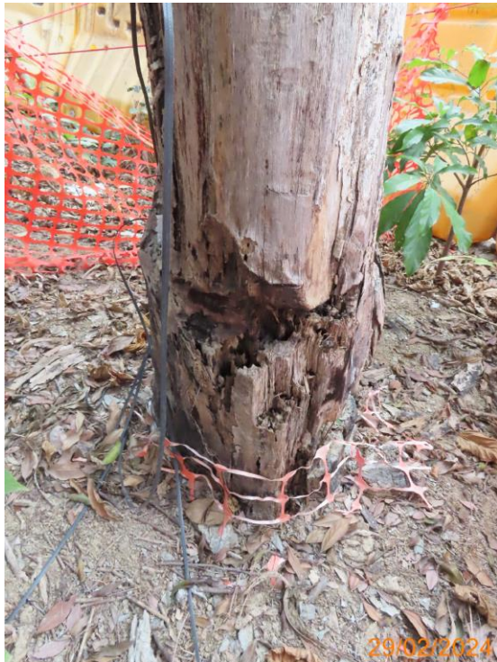
11: U041_Wood damage by termite
