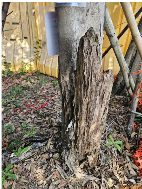
11: U041_Wood damage at trunk union#1
